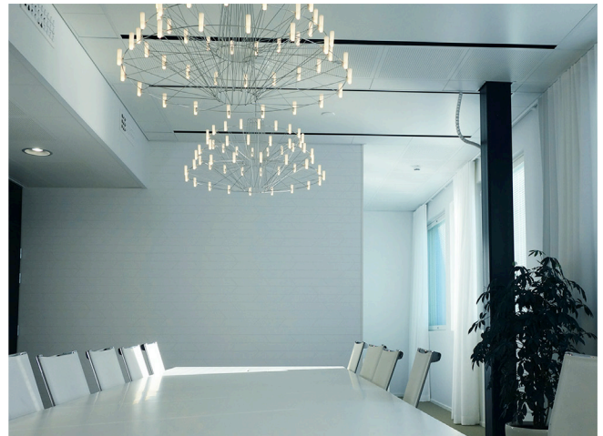
Panel integrerad i undertaket.
